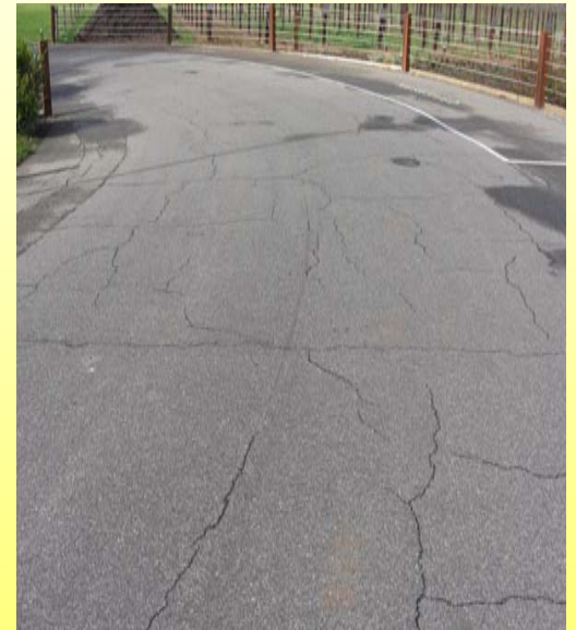
c. Fatigue Cracking
